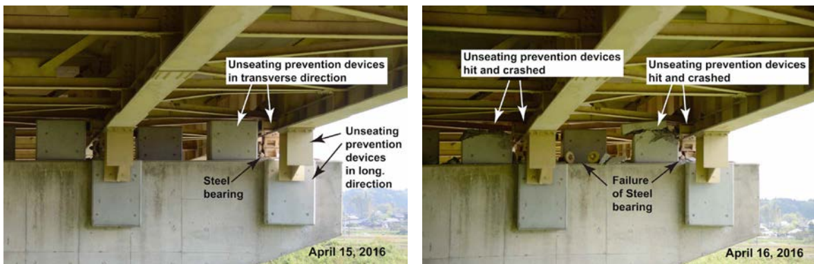
Fig. 6 – Unseating prevention device installed at Kiyamagawa Bridge, Kumamoto Prefecture, Japan, before (left) and after (right) the April 16, 2016, Kumamoto earthquake.
