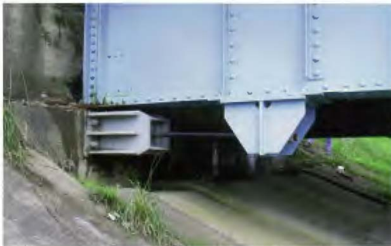
Fig. 5 – Unseating prevention device installed at Ono Bridge, Miyagi Prefecture, Japan, after the July 26, 2003, Northern Miyagi Prefecture earthquake [7, 8].
