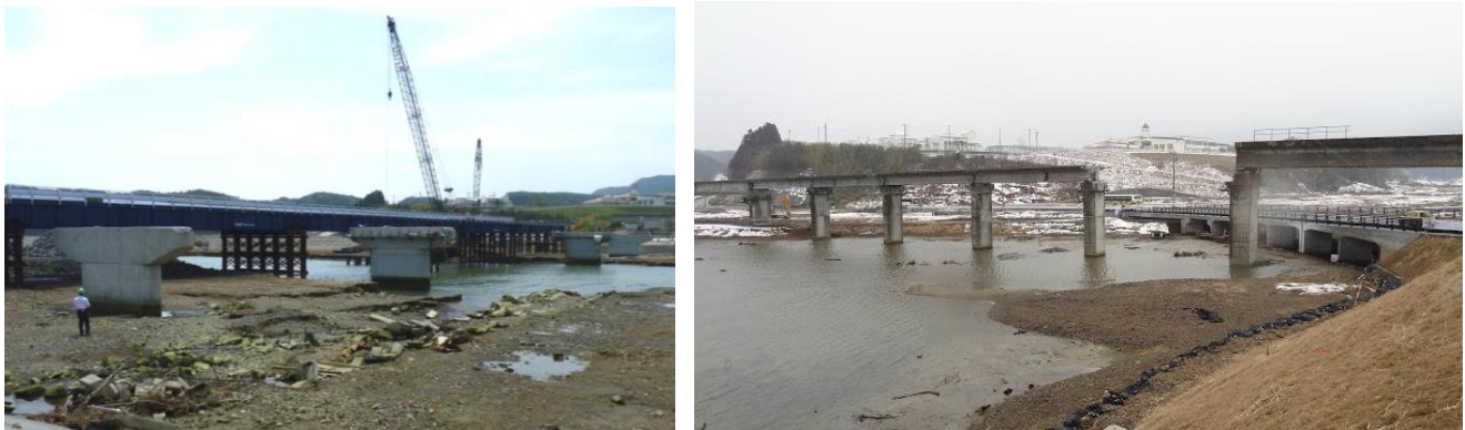
Fig. 1 – Damaged bridges after the 2011 tsunami in Japan: (a) Koizumi bridge on the left (from [1]) and (b) Tsuya railway bridge on the right (from [2])
