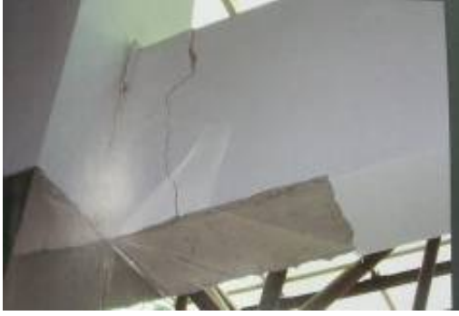
Fig.1 Crack of beam
