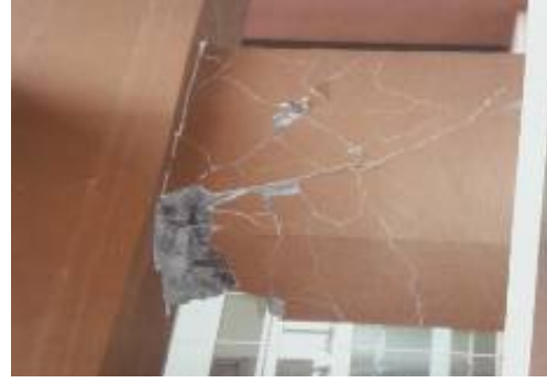
Fig.2 Spalling of beam
