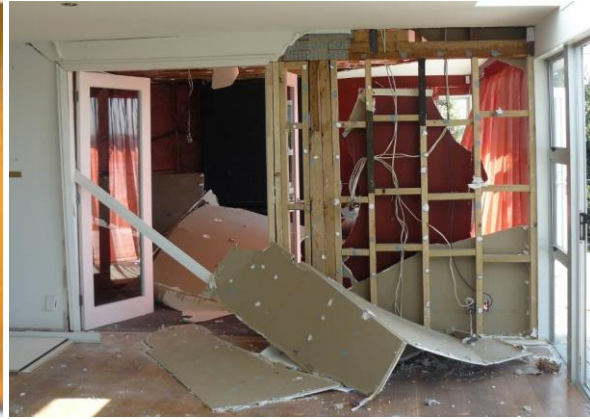
Fig. 2 – Failure of plasterboard internal linings.
