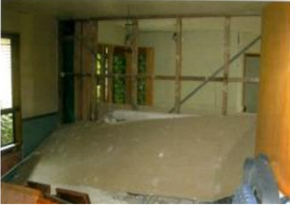
Fig. 1 – Failure of plasterboard/metal brace
