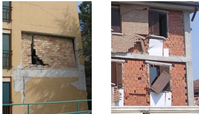
Fig. 1 – Observed damage to masonry infills in RC frame buildings following the a) 2009 L’Aquila (left) and b) 2012 Emilia earthquakes
