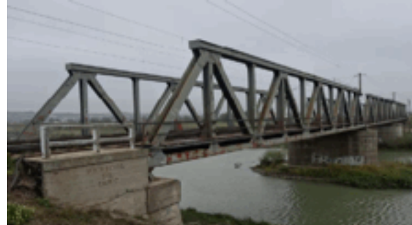
Case study: unseating of Siret River Bridge, Romania
