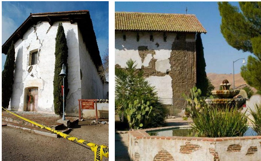
Fig. 9 (left) – Cracks in façade immediately following 2003 San Simeon earthquake [1]
