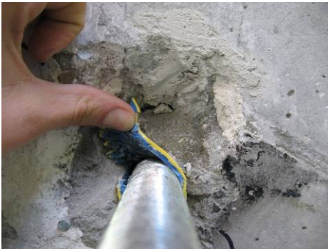
Fig. 7 - Rubber sheath deformation
