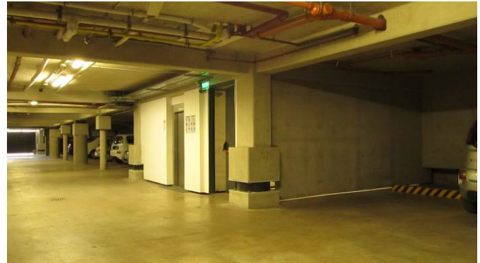
Figure 9: Isolators below the superstructure shear wall
