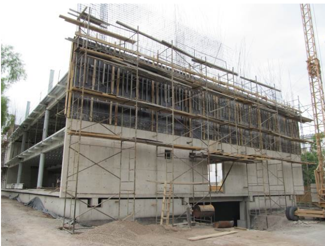
Figure 11: Basement perimeter, vertical gap
