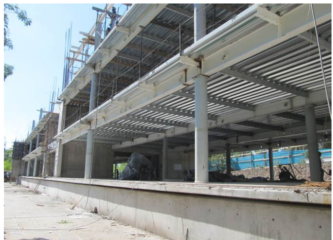
Figure 12: Basement perimeter, vertical gap
