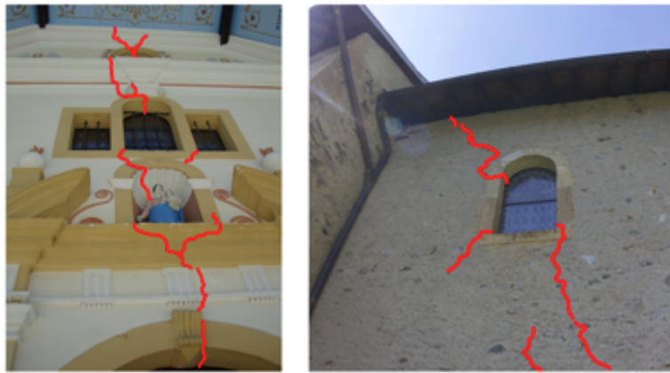
Fig. 9 Surveyed damages in NDG.
