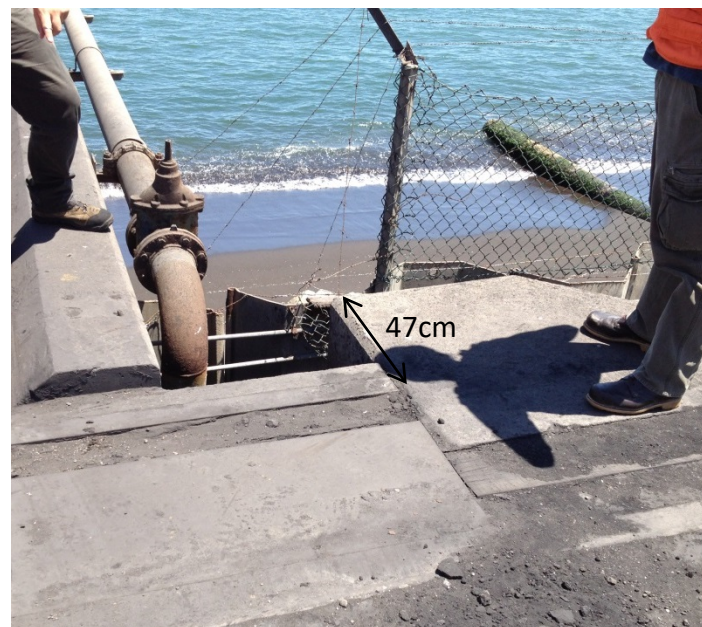
Figure 3 Displacement of ground relative to the South Pier
