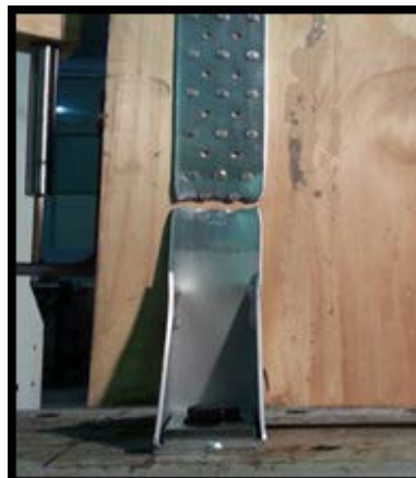
Figure 6 - Failure in a hold-down
