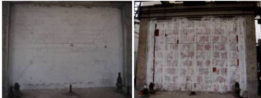
Fig. 14 – Out-of-plane tests. Cracking of the CIS and INSYSTEM 2 specimens at maximum deflection.
