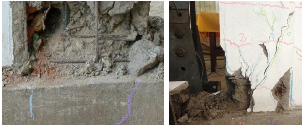
Fig. 10 – Crushing of the bottom of the columns for wall WV-1 (left) and wall WV-2 (right).
