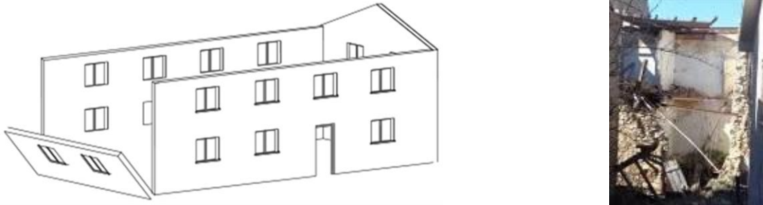
Fig. 8. Complete overturning of a perimeter wall in Sant'Eusanio Forconese
