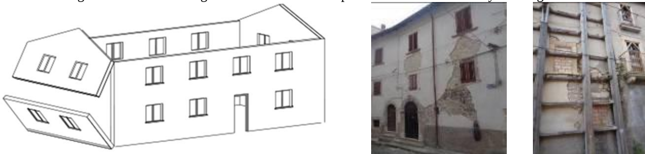
Fig. 10. Out-of-plane flexural mechanisms of the external leaf of a perimeter wall equipped with iron ties of a masonry building in Castelvechio Subequo
