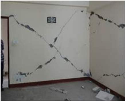
Fig. 6 – Shear failure in infill brick walls (KM)
