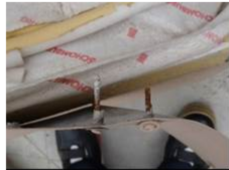
Fig. 13 – Screws connecting the joint cover and RC frame (KD)
