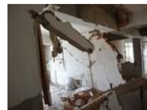
(c) Interior damage (3F)
