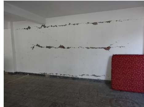
Fig. 7 – Cracks along brick joints (KM)
