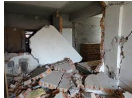
Fig. 9 – Brick wall collapse (KP)
