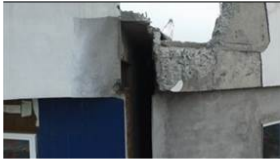
Fig. 15 – Damaged parapet of Building KE
