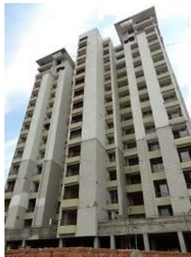
(a) Exterior damage
