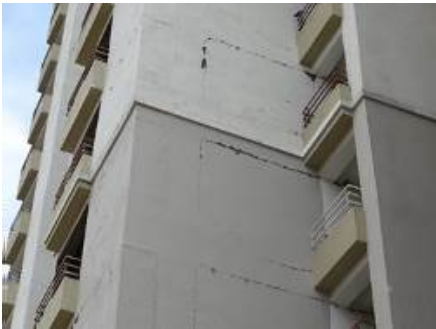
Fig. 8 – Cracks along joints between brick wall and RC frame (KP)
