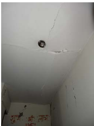
Fig. 10 – Ceiling damage (KD)
