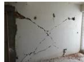
(b) Interior damage (11F)
