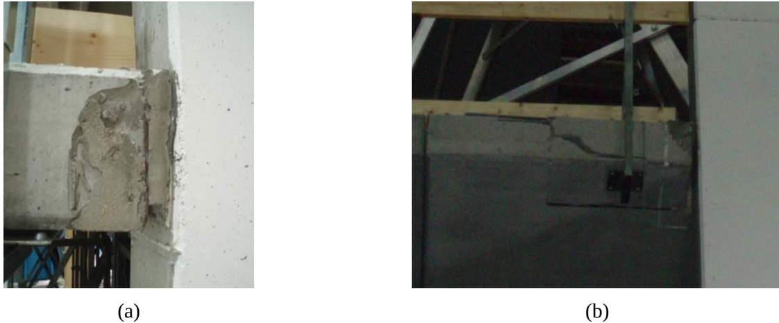
Fig. 11 – Detail of one beam-to-wall simply grouted connection (a) spalling at the end of the test with PGA equal to 0,15g and (b) failure at the end of the test with PGA equal to 0,30g
