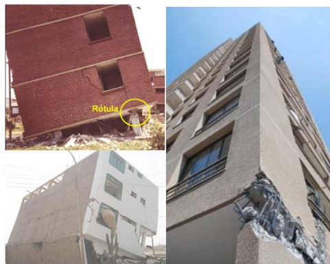
Fig. 3 - Structural failures at the first story columns due to a soft story configuration [6]
