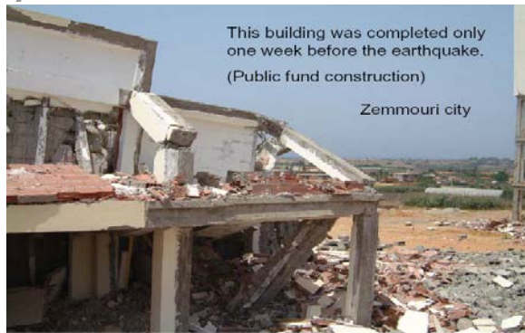
Fig. 5 – Bad concrete recast And execution (Boumerdes 2003 Earthquake)
