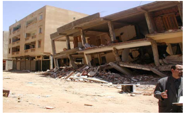
Fig. 6 – Soft story and bad execution (Boumerdes 2003 earthquake)
