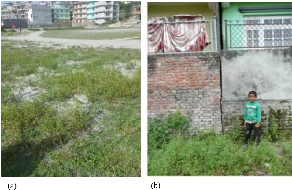
Fig. 10 – (a) Large sand boils of fine sand in Manamaiju (b) Tilting of building due to lateral spreading in Manamaiju
