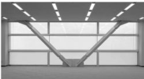
Photo 2 – Steel Damper in Long Direction
