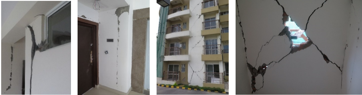
Fig. 3 – Observed damaged in (a) corner of infill wall, (b) beam corner, (c) exterior, d) interior/exterior wall
