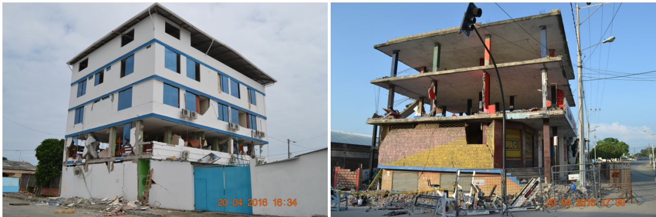
Fig. 4 – Multistory R.C. buildings with flat slabs that were damaged during the 2016 Ecuador earthquake
