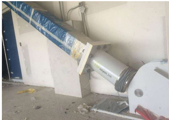
Fig. 11: Instrumented damper in the building.
