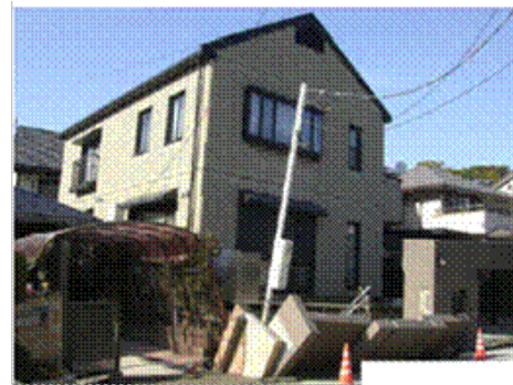
Phot.3 Damage to a residential house in Urayasu due to liquefaction during the earthquake.
