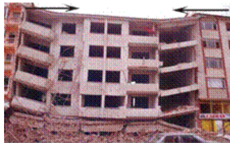
Fig.1- Two buildings pounded to middle building because of deficient separation space during Marmara earthquake (1999) in Sakarya, Turkey [7]
