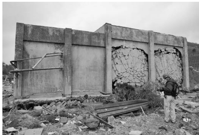
Fig. 1 – An example photo of destruction of RC outer wall
