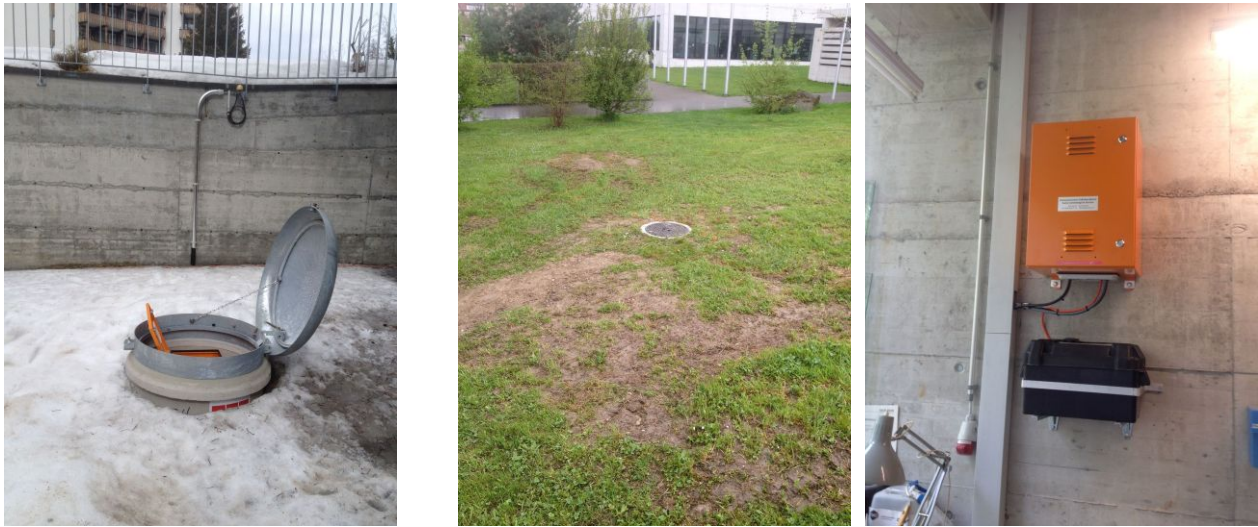
Fig. 4 – Left: Station SDAK in Davos (large vault). The GPS antenna and the antenna for the mobile telephone network for the data transmission are fixed at the wall behind the station. Center and right: Station SKRK in Kreuzlingen is installed in a small vault. The communications and power hub with the data logger is installed in a building nearby (orange box). The black box is the emergency battery.
