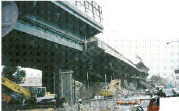
(a) at 1995 Kobe Earthquake
