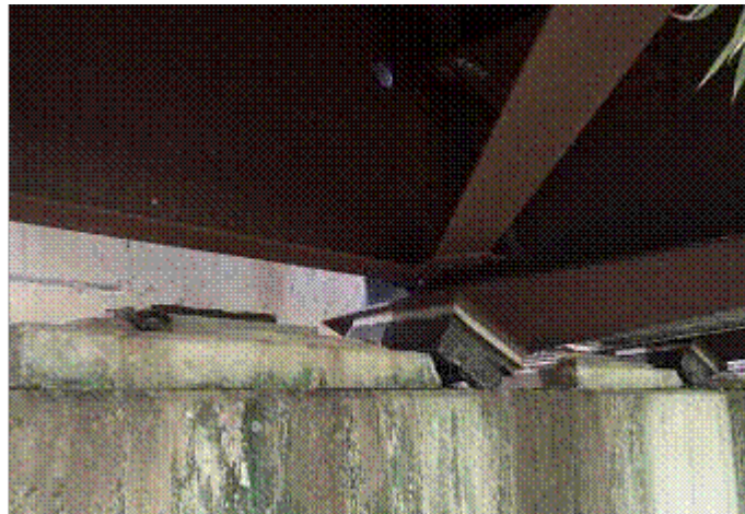
Fig.18 Bearing damage at Okirihata Bridge.
