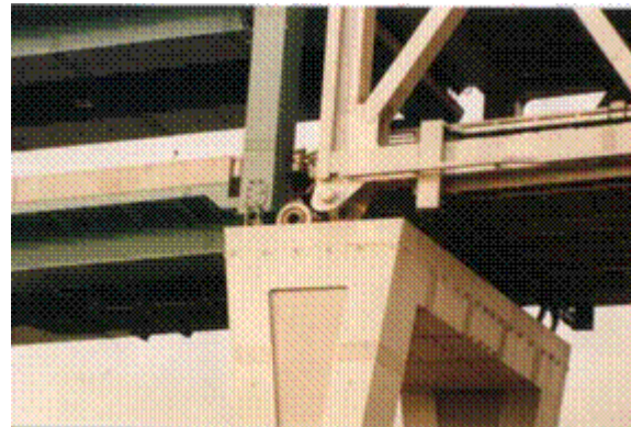
(b) damage at 1995 Kobe Earthquake
