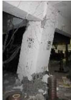
(b) Damaged column (X2Y4)
