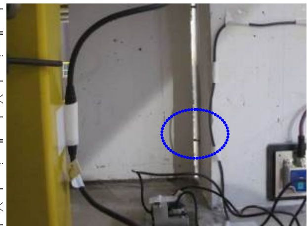
Photo 1 – Gap and Joint Bar
