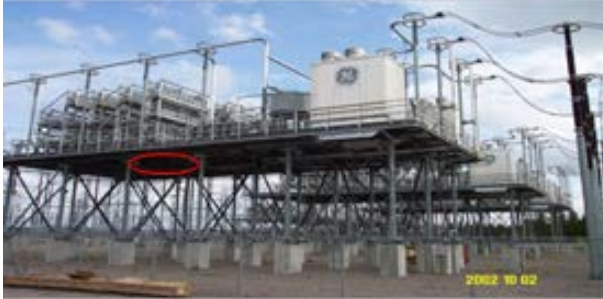
Fig.24 – Capacitor bank platform
