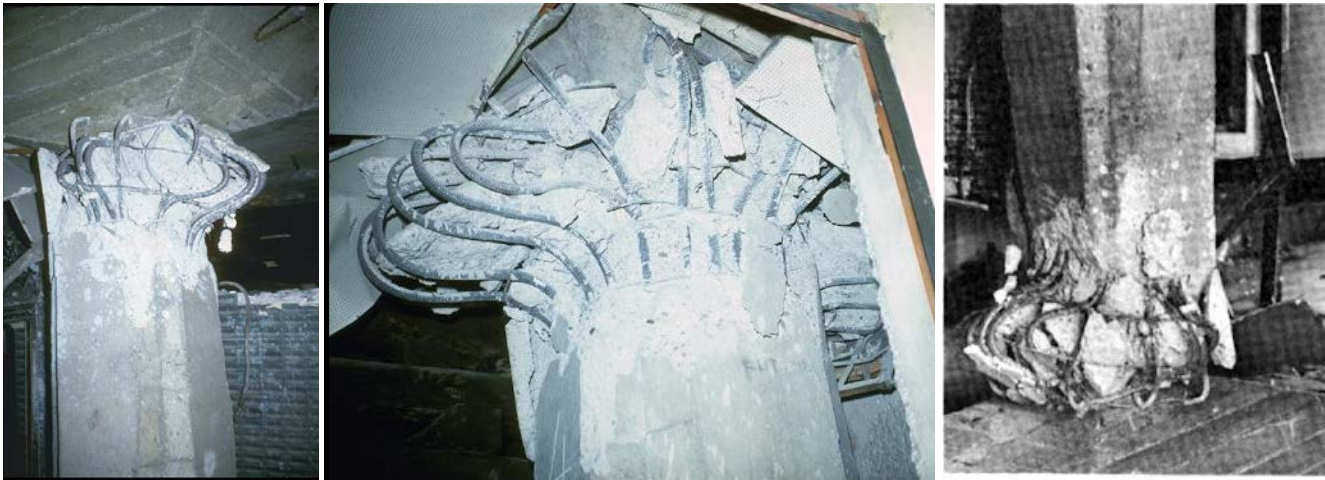
Fig. 3 – Ground story top and bottom column failures (EERI collection)
