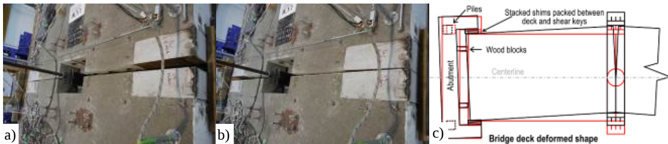
Fig. 12: a) Deck-deck gap opening at 2% drift test 1 during the push cycle (left) and pull cycle (right). b) Plan view of deformed bridge shape (black lines).
