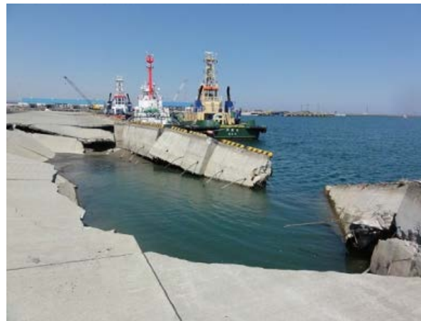
Photo 1– Damage to Quay 1-4
