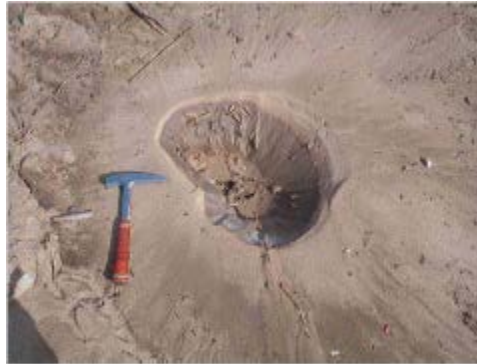
Fig. 7 – Observed liquefaction near the Sebaou Bridge
